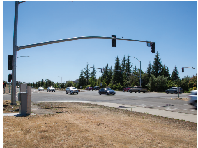
TSP installation, Folsom CA
